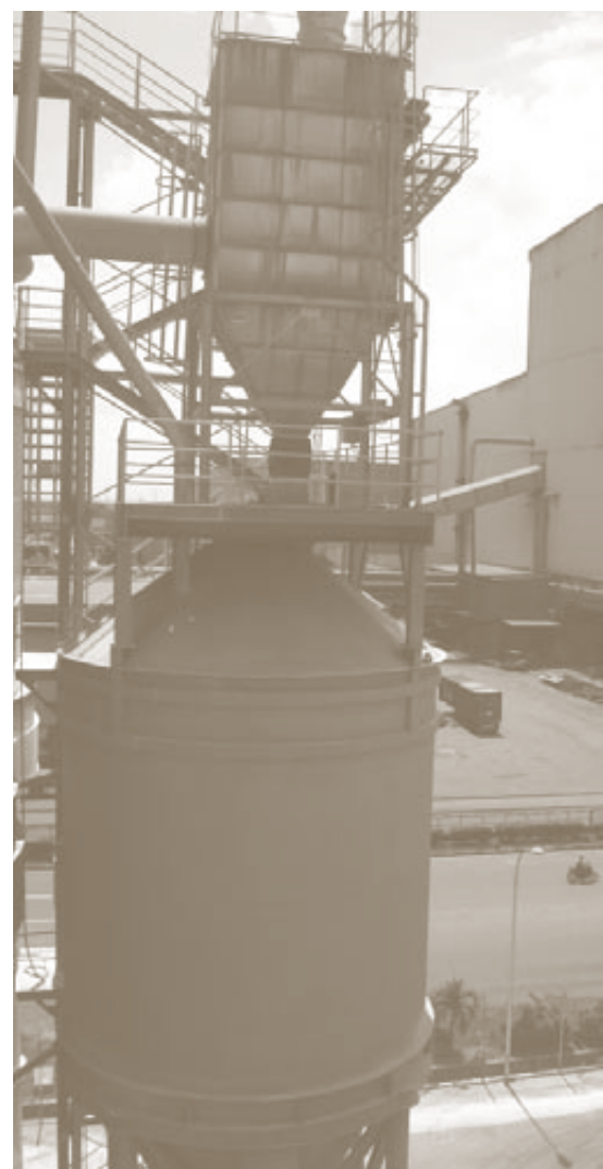
Quicklime fine silo and silo dust collector
